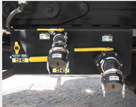
3" High Volume Plumbing With Labeled Controls
